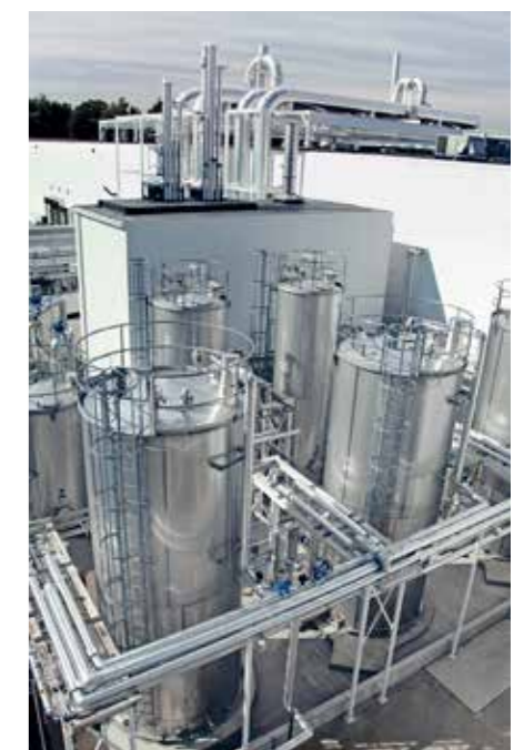
Solvent distillation column and tank farm
