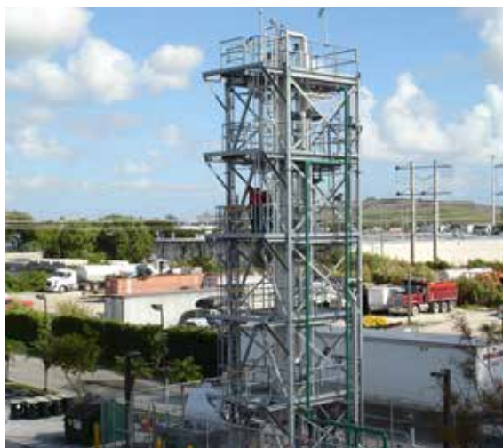
Distillation system at pharmaceutical plant
