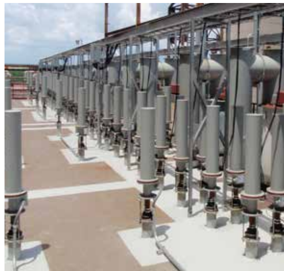
Wet and Dry Precipitator Upgrades/Rebuilds
