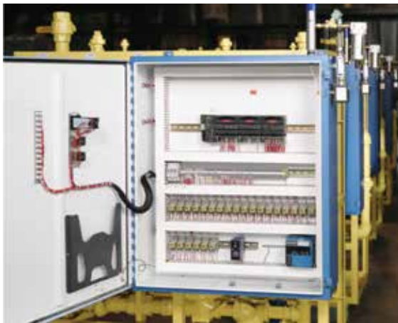
Burner Management Systems
