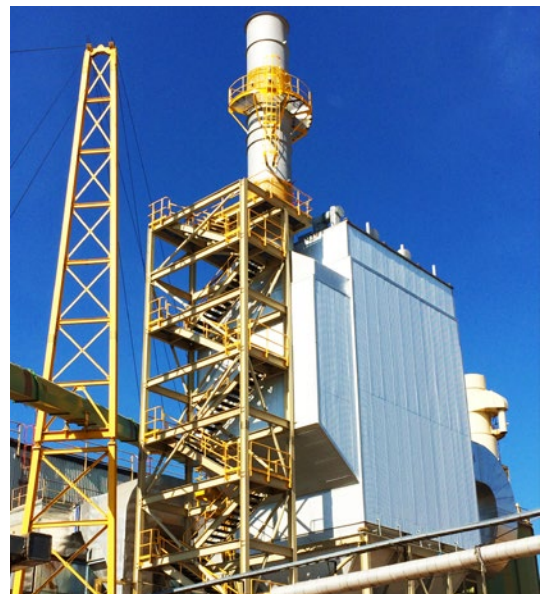
Proven process knowledge thanks to multiple installations
