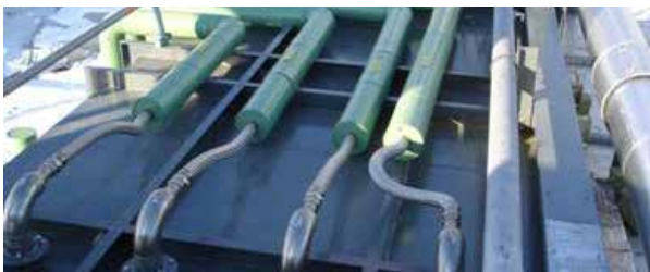
Injection of fluid streams into RTO combustion chamber
