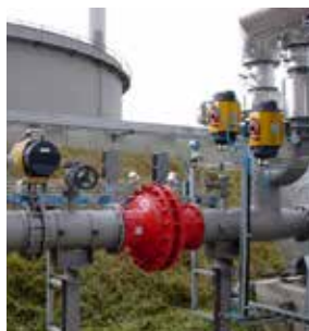
Detonation arrestor and double shut-off valves
