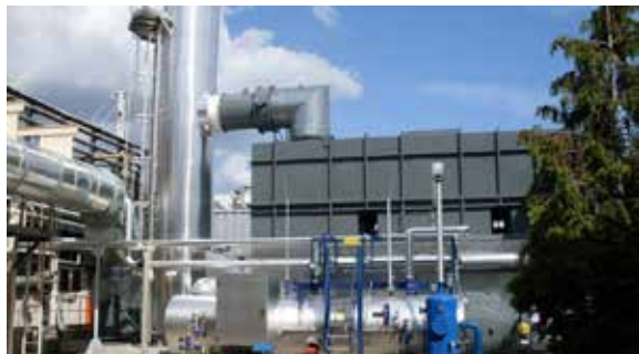
RTO with heat recovery for steam generation
