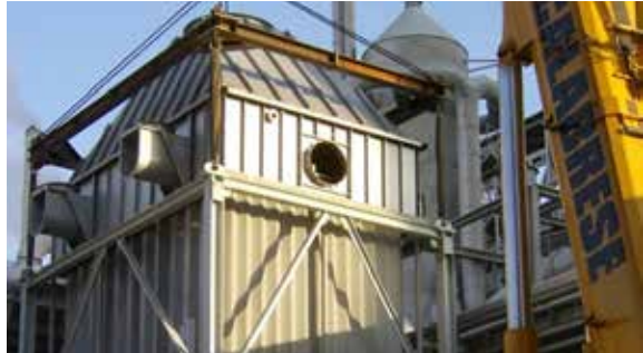
WESP for particulate control from calcining kiln
