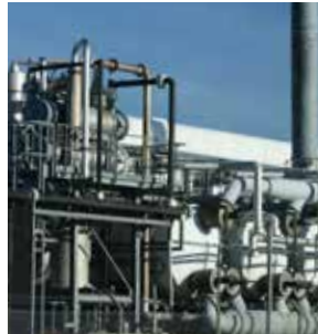
Solvent recovery plant recovering 440 lb/hr (200 kg/hr) of dichloromethane from 18,500 SCFM (440 Nm 3 /hr)
