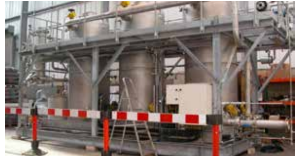
Adsorption skid to recover HFCs and CFCs from aeration tanks
