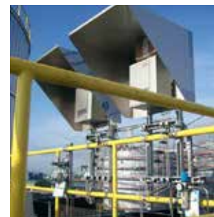
Redundant VOC concentration level control
