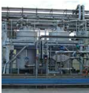
Duty and stand-by adsorbers for mixed VOCs from batch manufacturing plant
