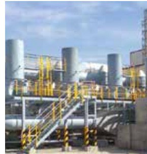
Toluene recovery plant handling 222,000 SCFM (350,000 Nm 3 /h) and 5,500 lb/hr (2,500 kg/hr)
