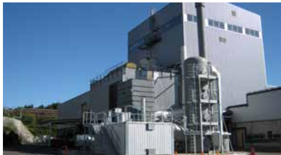
RTO and tail gas HCl scrubber
