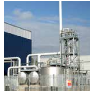
Acetone recovery plant recovering 330 lb/hr (150 kg/hr) from 5,100 SCFM (8,000 Nm 3 /hr) including distillation
